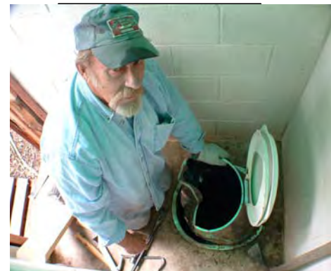
If you need a toilet repaired, DO NOT call Clint Tawse! Seriously, Clint got the unenviable job of removing this stuck commode...the hard way.
